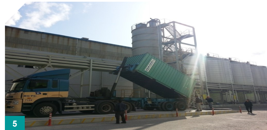
5 ASIA PAPER Starch Power Unloading System
