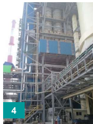
3 HAN GLASS Petro Coke Handling System
