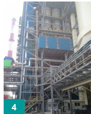
3 GE4 Limestone Handling System
